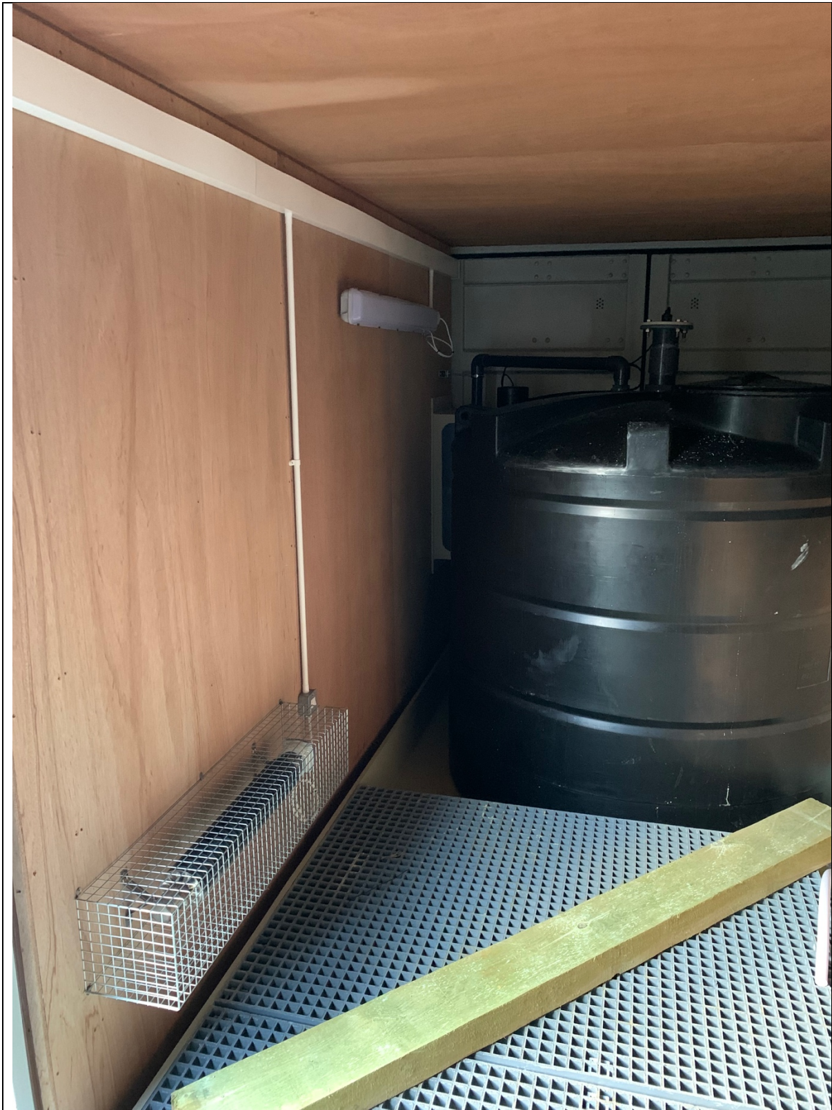
GRP Flooring on PP bund + 1kW Heater
