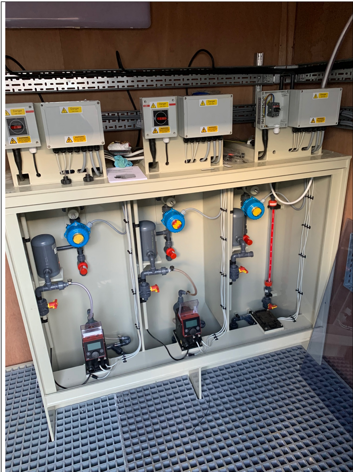
Duty/Standby + Manual Dosing Pump Skid (RHS pump missing)
