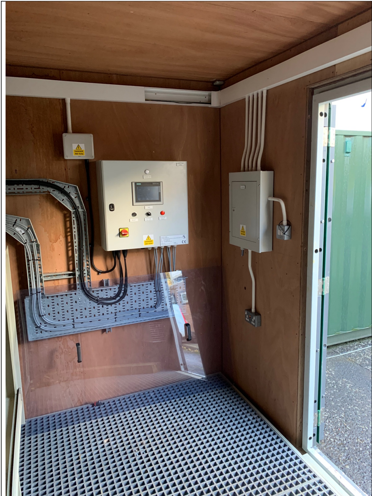
PLC + HMI Local Control Panel * Container Domestic Dis. Board
