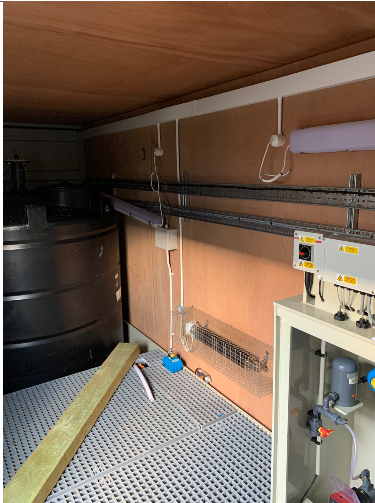
GRP Flooring on PP bund + 1kW Heater
