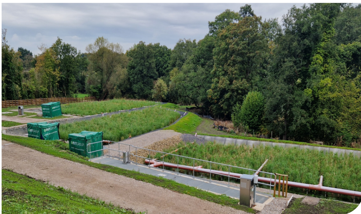
Photograph of the ARMStorm™ CSO wetland treatment system.
