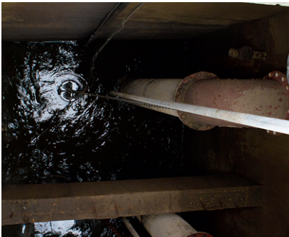
Inside a Sanepar lifting station
